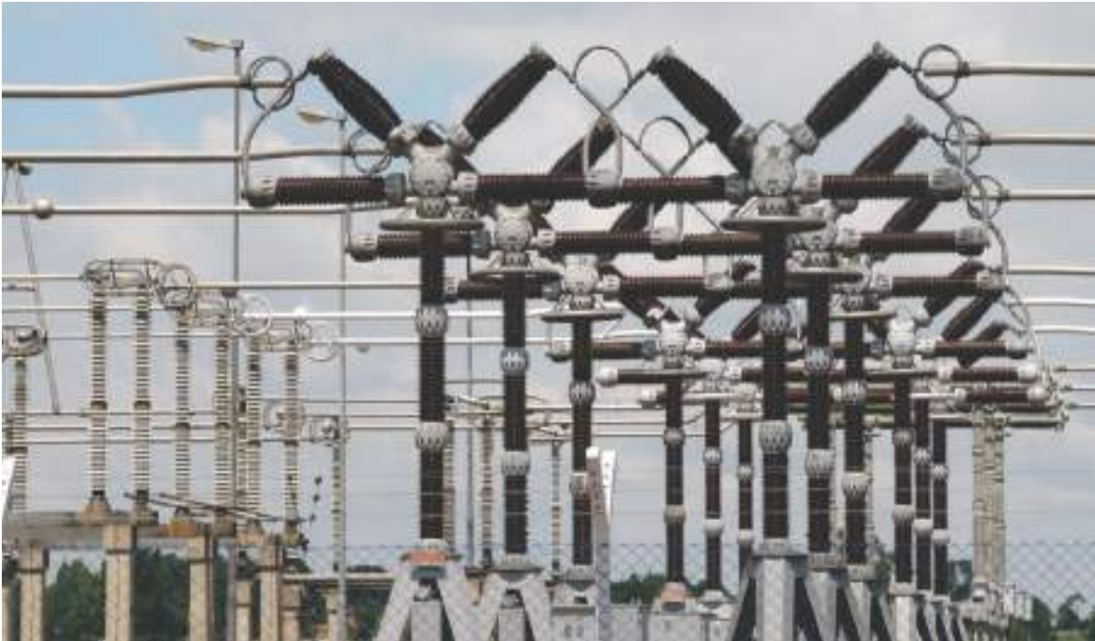
■ Power Sub-Station, Abuja.
